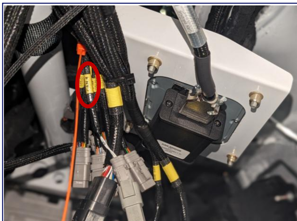
VBOX Wiring Labeled "CAN4" Underneath Dash
